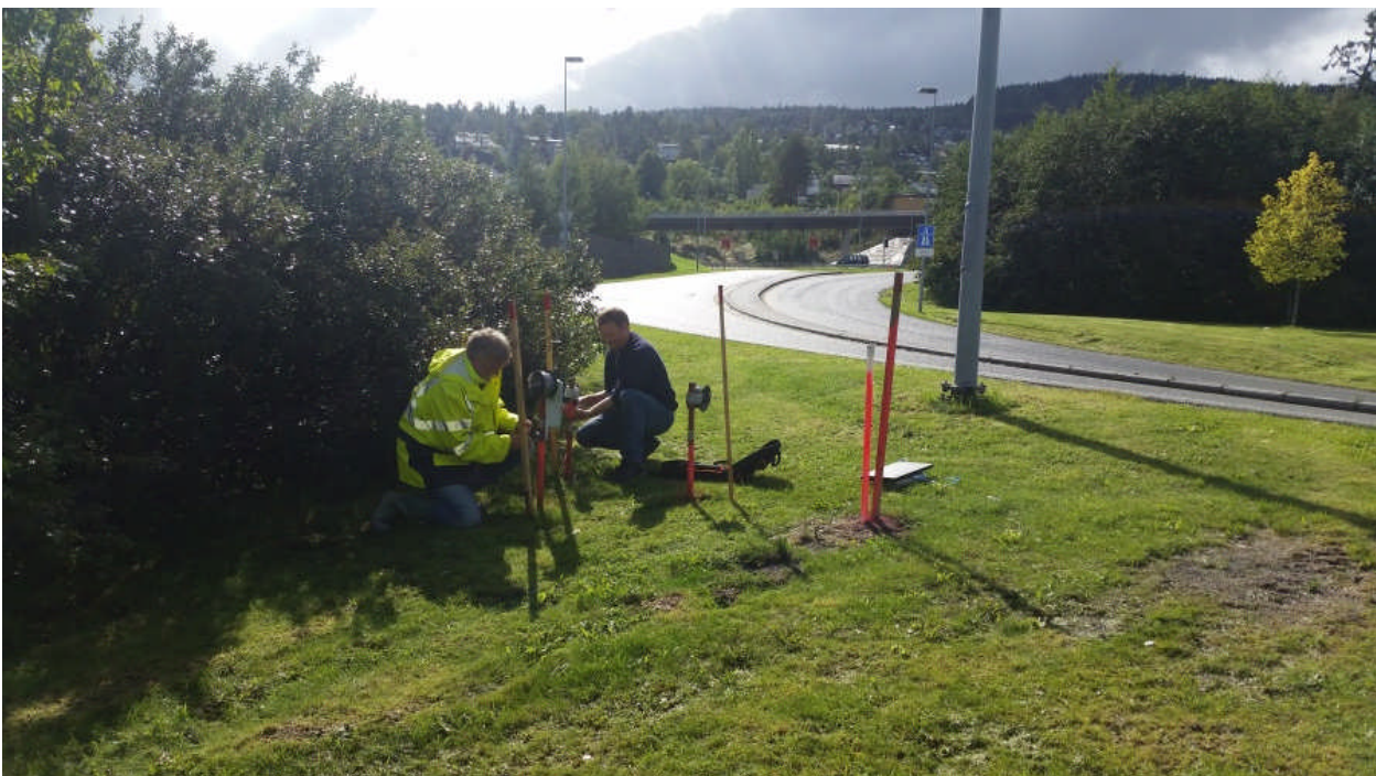
Fig. 1 – Remote read-out solution example: Monitoring of pore pressure in clay at different depths under a road. The gateway receives settings and sends logged data via the mobile phone network.
